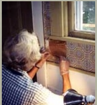
Stencils from the 19thc and earlier were formed of copper (above), vellum or parchment cut by hand. Here the stencil is taped to the wall as the color it represents is about to be applied.
