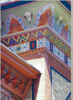
High Victorian stencils (above) on the exterior of Olana, the home of artist Frederick Edwin Church, overlooking the Hudson, 1870-90
