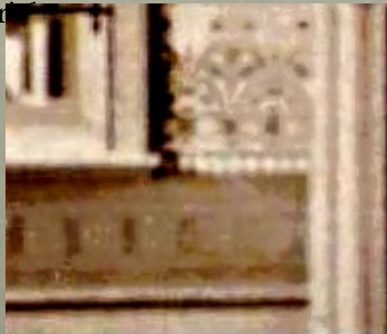
Detail of stencil band we have uncovered and are recreating between top of stringcourse and bottom of sill. Note second band up; it's floral. (detail above from 1884 photo to right)
